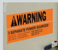
Equipment and panel labeling
